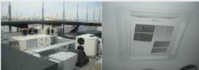
Escala Yacht Club – Heat pumps start up on the roof and cassette type terminals
