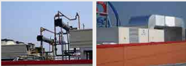
Caselle Center – Recovery from food refrigeration and water-to-air Rooftop for malls
